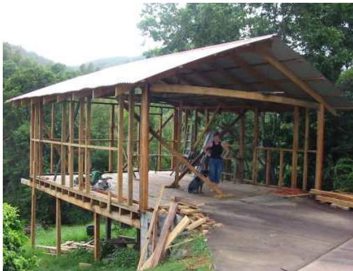
Figure 3. Some of the sawn timber in a car port still at the framing stage
